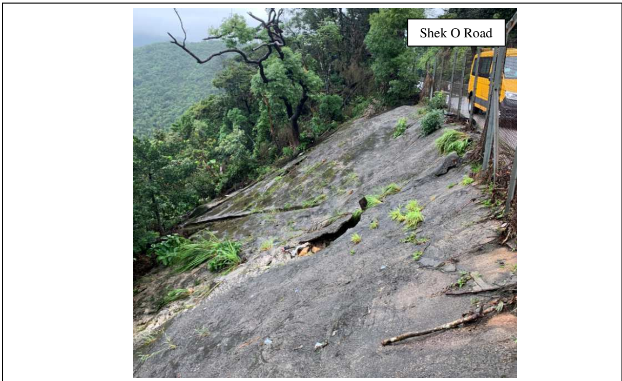
Figure 5.8 Cracked Shotcrete Cover on Slope No. 11SE-D/F174 (Photograph Taken on 9 September 2023)
