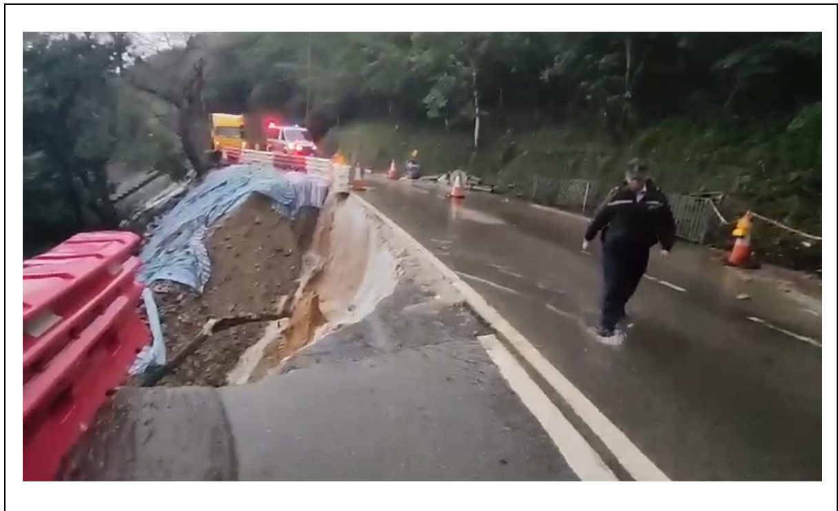
Figure 5.15 Significant Overland Flow from Shek O Road towards the Fill Slope (Photograph Taken on 14 September 2023)
