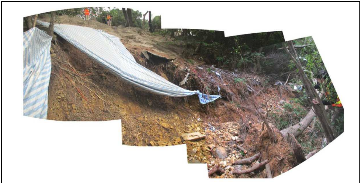
Figure 3.4 The 2016 Landslide (Photograph Taken on 29 November 2016)
