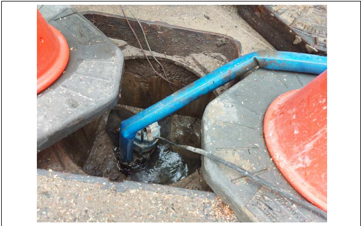
Figure 5.17 Blocked Roadside Gully on Lay-by Area (Photograph Taken on 14 September 2023)
