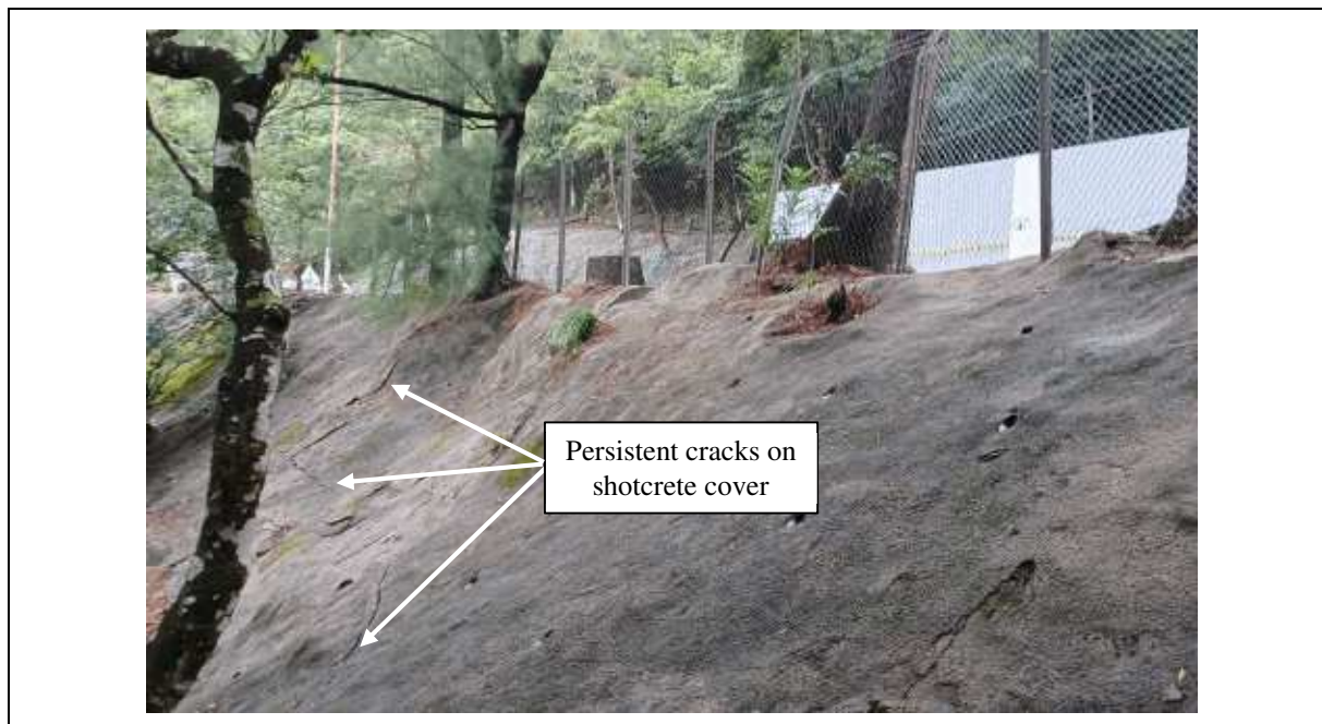
Figure 3.5 Surface Condition of Slope No. 11SE-D/F47 after Maintenance Works (Photograph Taken on 4 November 2022)
