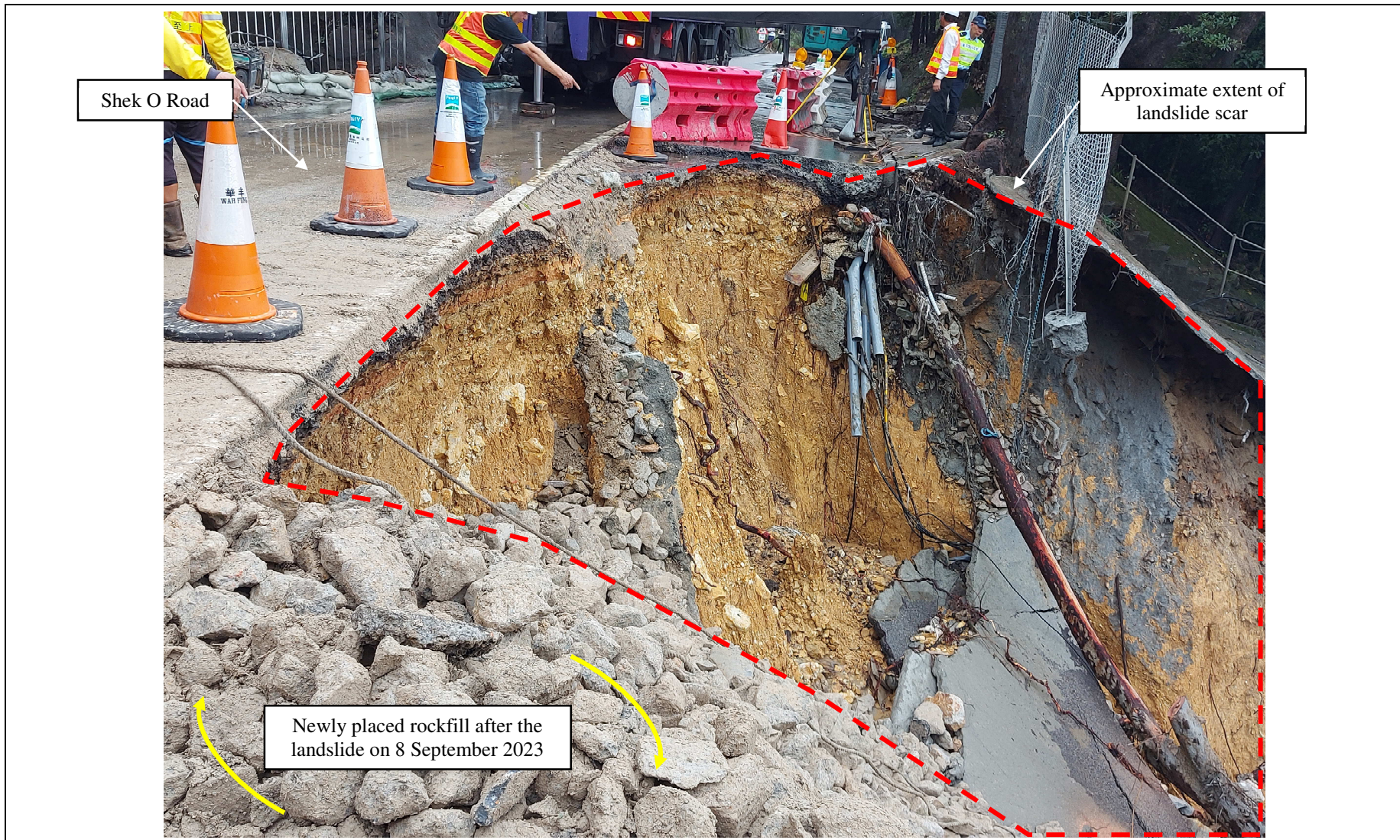
Figure 1.3 General View of the Landslide on 14 September 2023 (Photograph Taken on 14 September 2023)
