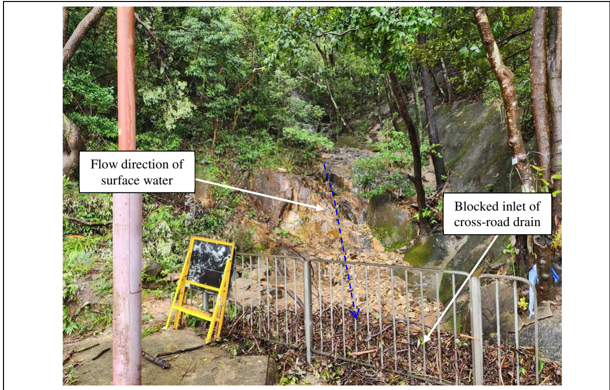
Figure 5.5 Blocked Catchpit of the Upslope Rocky Natural Stream Course (Photograph Taken on 9 September 2023)
