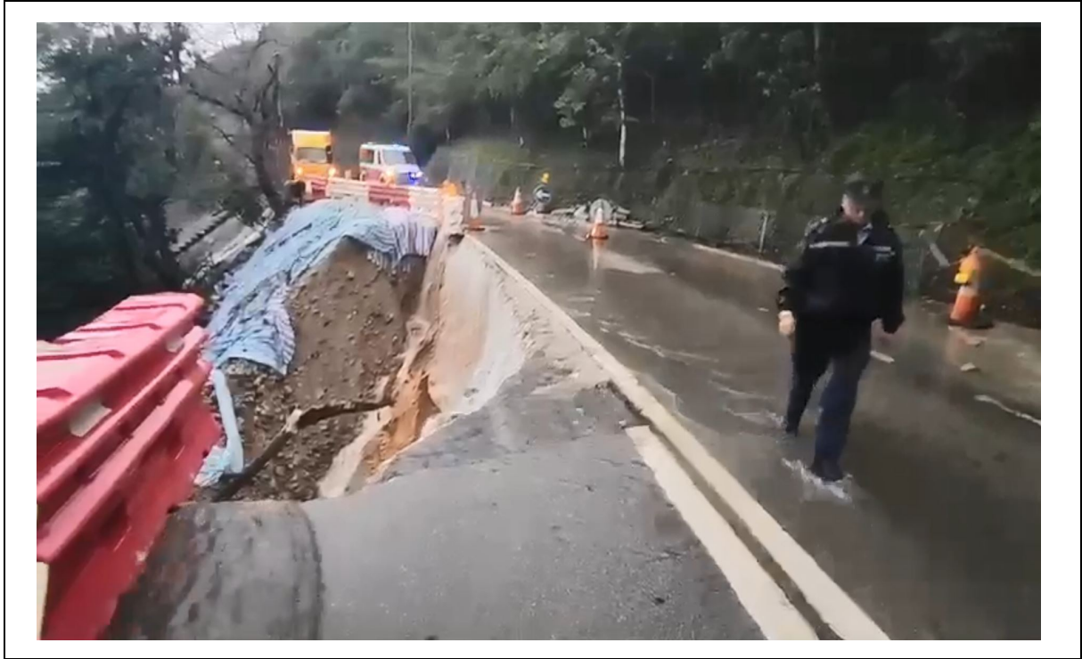
Video B1 Video Clip showing Overland Flow from Shek O Road towards the Fill Slope (Video recorded on 14 September 2023)
