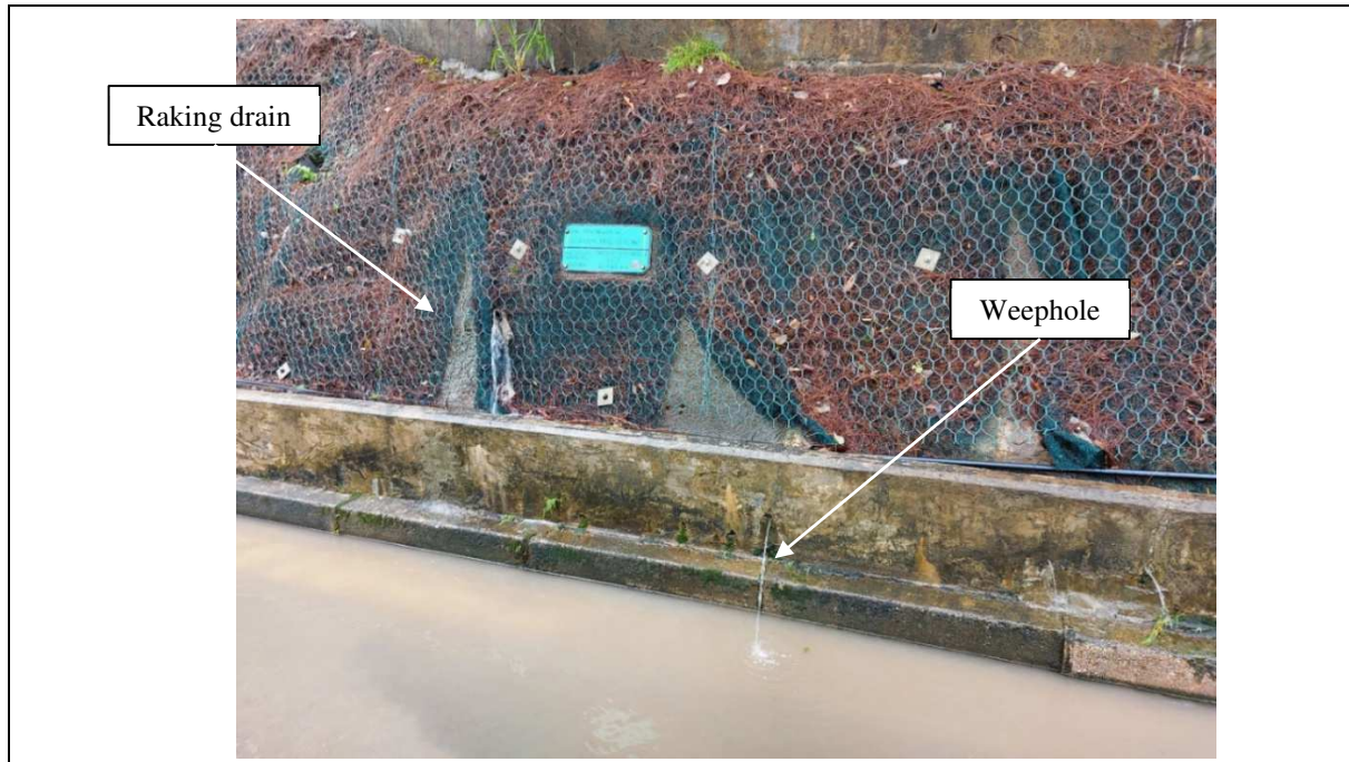
Figure 5.18 Persistent Water Flow on Nearby Cut Slopes (Photograph Taken on 14 September 2023)
