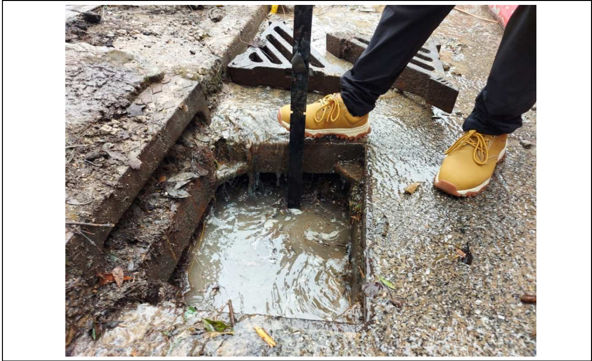
Figure 5.16 Blocked Roadside Gully on Shek O Road (Photograph Taken on 14 September 2023)
