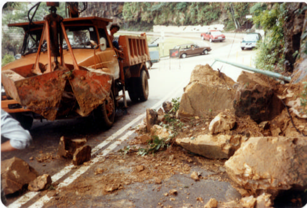
Plate 22 Rock cut slope failure at junction of May Road & Magazine Gap Road. (Incident No. HK 84)
