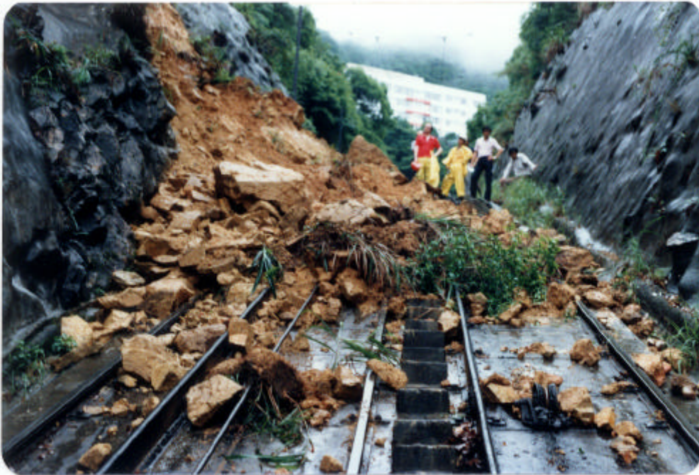
Plate 21 soil/rock cut slope failure at Tramway near May Road Station. (Incident No. HK 6)
