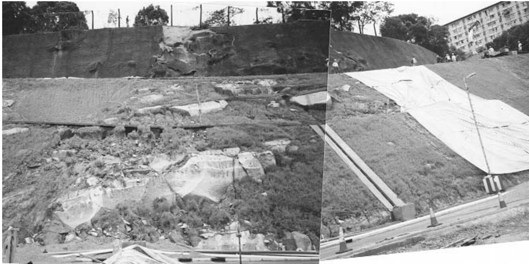
Plate 3 – View of the Site the Day After the Landslide (Photograph Taken on 10 June 1998)
