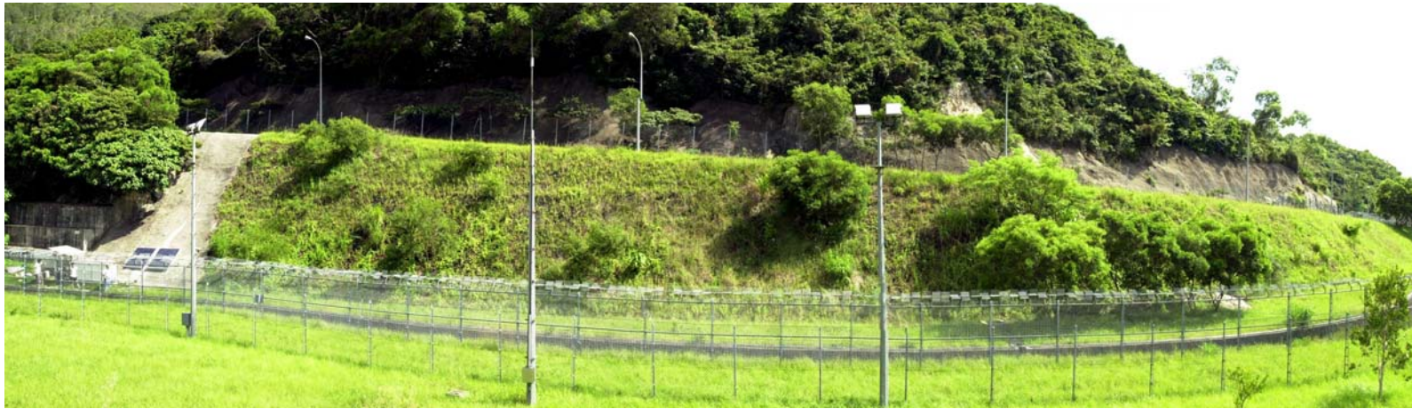
Plate 9 - General View of the Slope with the Installations of the System Components
