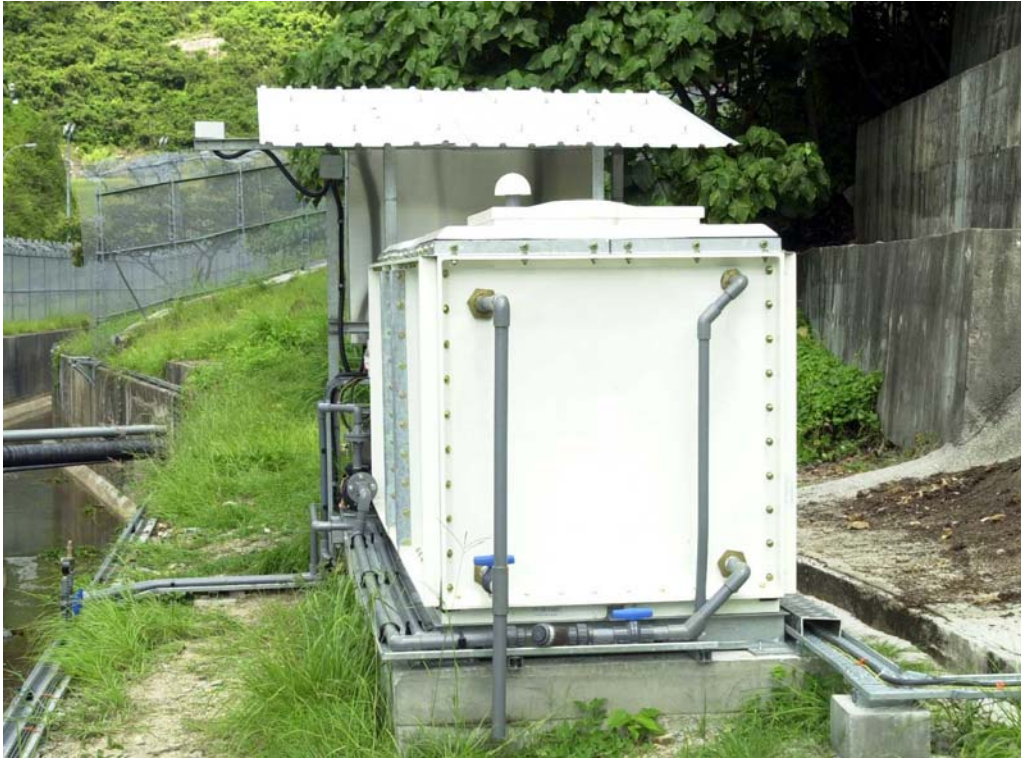
Plate 6 - Water Storage Tank of the System
