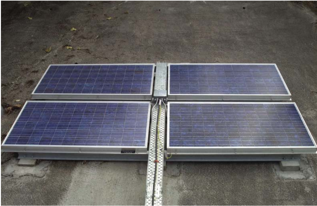
Plate 2 - Photovoltaic Panels of the System
