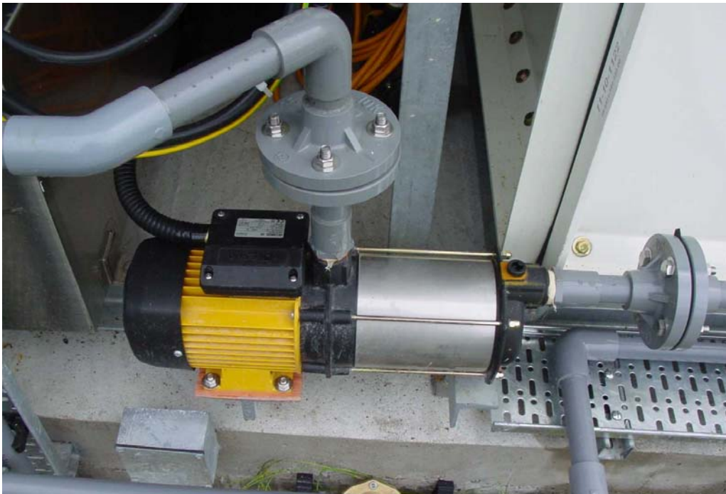
Plate 7 - Irrigation Pump of the System
