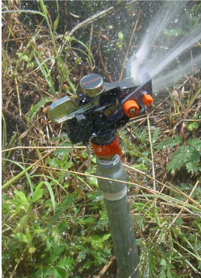
Plate 8 - Sprinkler of the System
