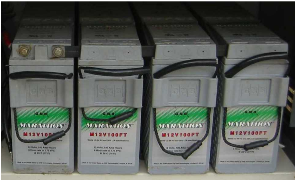
Plate 3 - Rechargeable Batteries of the System
