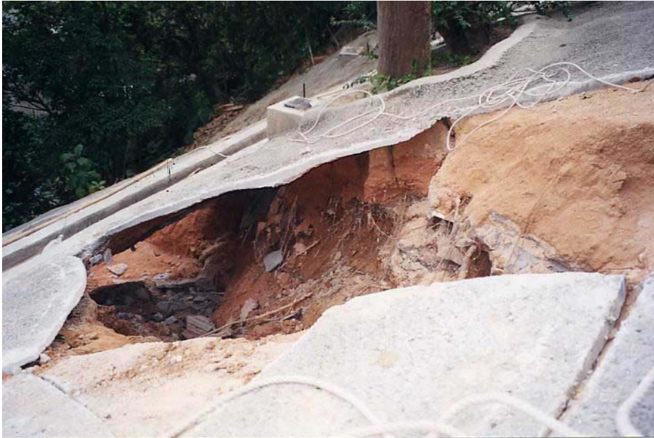
Plate 13 - Washout of Soil from underneath the Shotcrete Cover - Pokfield Road (Photograph taken on 4 February 2002)
