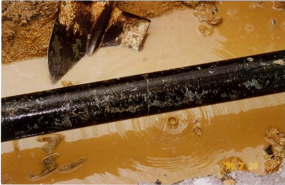
Plate 17 - Leakage Identified from a 75 mm Diameter Galvanized Iron Fire Services Pipe at the Crest of the Slope - Chinese University (Photograph taken on 6 July 1999)
