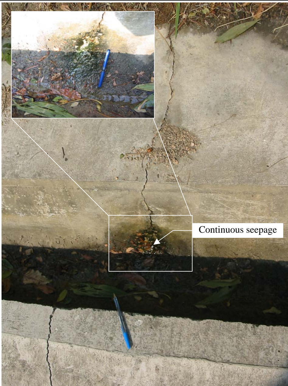
Plate 31 - Continuous Seepage at Cracked Surface Channel - Tai Po Road (Photograph taken on 6 January 2005)
