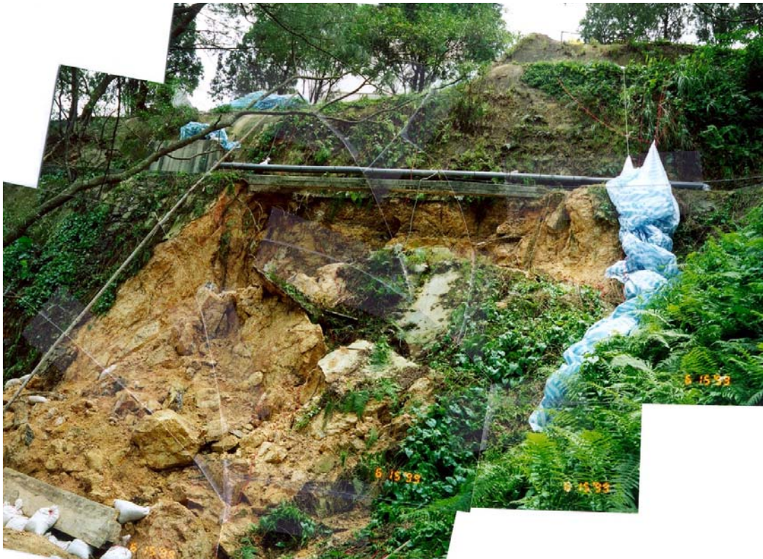
Plate 16 - General View of the Landslide - Chinese University (Photograph taken on 15 June 1999)
