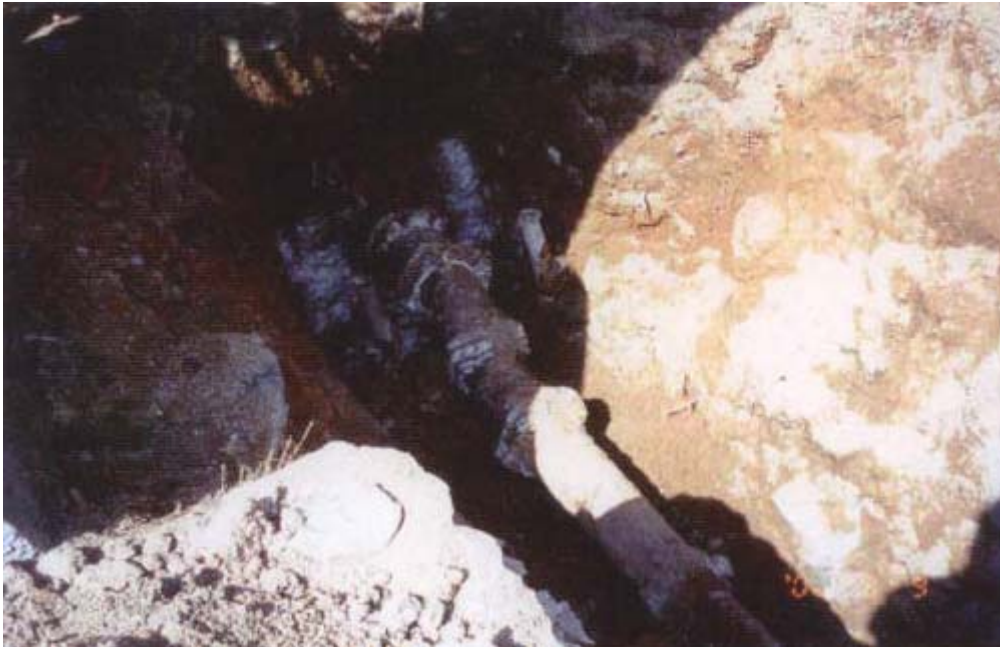
Plate 10 - The 150 mm Heavily Corroded Water Pipe near the Footpath at Slope Toe - Lai Chi Kok Hospital (Photograph taken on 9 September 2000)
