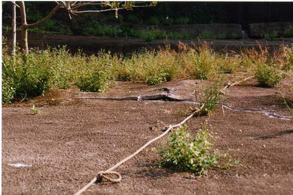
Plate 6 - Downslope View of the Zone of Bulging at Upper Batter - Hiu Kwong Street (Photograph taken on 5 May 1998)
