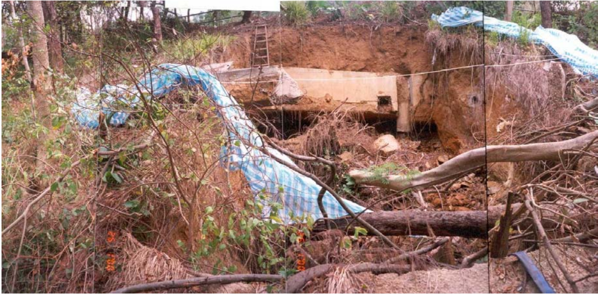
Plate 7 - View of Main Scar and the Leakage Collection Trough - Kau Wah Keng Village (Photograph taken on 26 January 2000)
