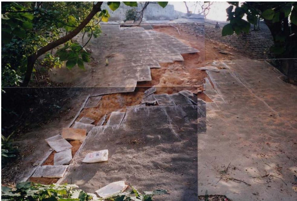
Plate 14 - View of the Erosion Gully After Removing the Shotcrete Cover - Pokfield Road (Photograph taken on 25 February 2002)
