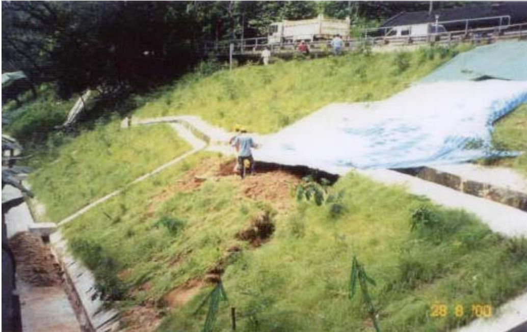
Plate 9 - General View of the Landslide Scar - Lai Chi Kok Hospital (Photograph taken on 28 August 2000)
