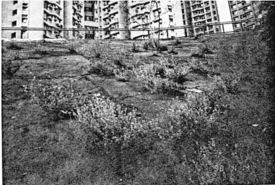
Plate 5 - View of the Zone of Cracking and Bulging in Shotcrete - Hiu Kwong Street (Photograph taken on 14 April 1998)
