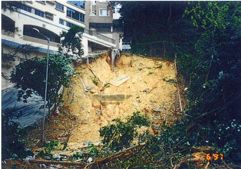
Plate 24 - General View of the Landslide - Chung Shan Terrace (Photograph taken on 5 June 1997)
