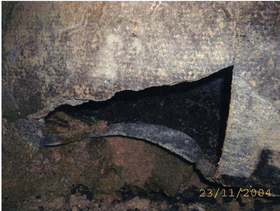
Plate 29 - Close-up View of Broken Saltwater Main - Sau Mau Ping (Photograph taken on 23 November 2004)
