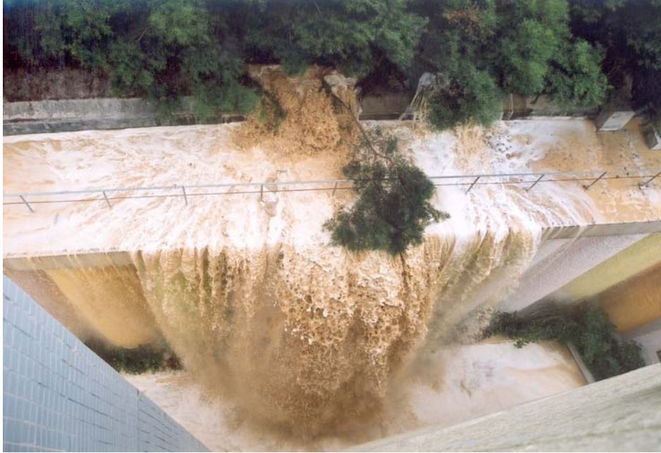
Plate 27 - General View of Muddy Water Discharging from Slope No. 11NE-D/CR15 - Sau Mau Ping (Photograph taken on 23 November 2004)
