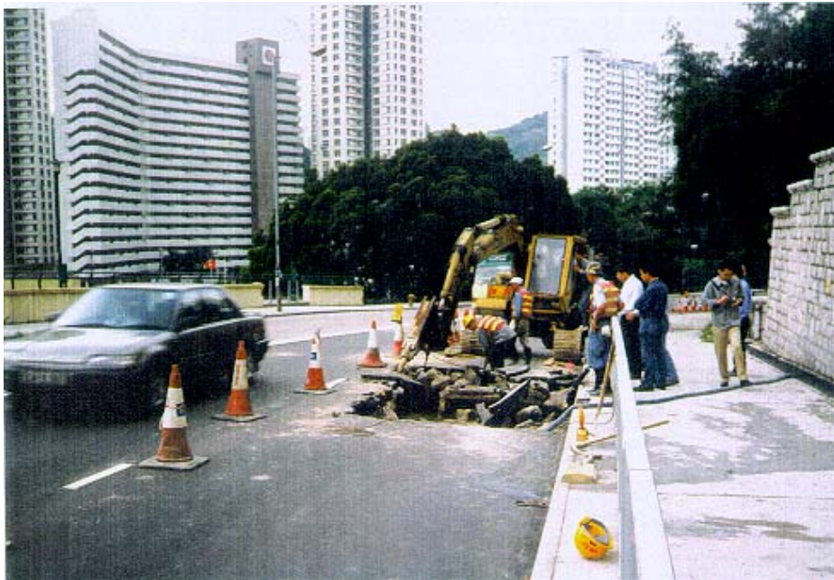
Plate 4 - View of Exploratory Pit Opened at the Location of Leak in Water Main along Northern Side of Hiu Kwong Street (Note blue hose for de-watering. Photograph taken on 14 April 1998)
